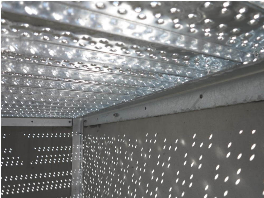
Figure 4. Fire protection gratings resting on angle bars.
